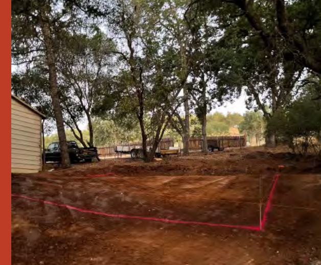
Ramey built the studio with help from his friend Rich Cummings and support from his wife Erin. Above, the first steps toward its construction; below, the structure takes shape.
